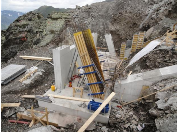
Connection of 4 single foundations with beams in order to exclude differential deformations between foundations
