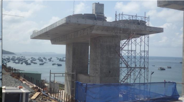
Drive station near seaside
