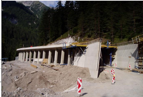
Avalanche protection of road and walkway
