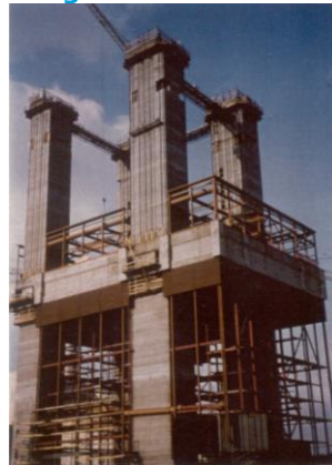
Complete design on behalf of Siemens Austria Lifting of head truss (10.000 tons) up to 76m height
