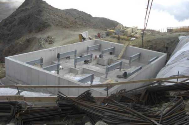
Tower 3: Tank below foundation
