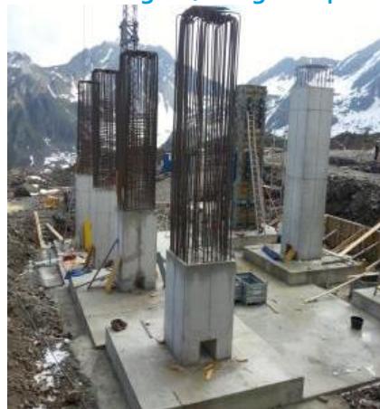
3S-MGD Pardatschgrat / Ischgl – Top station
