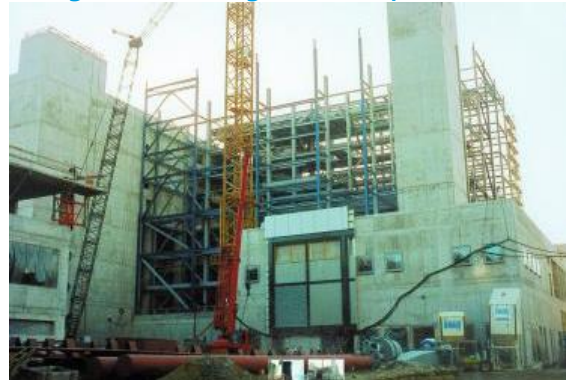
Böblingen – REA Co-generation plant
